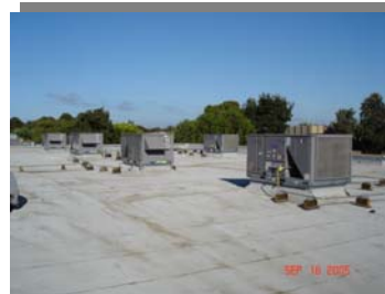
Completed the roof replacement and installation of new HVAC package units at Oak Grove, Building U.
